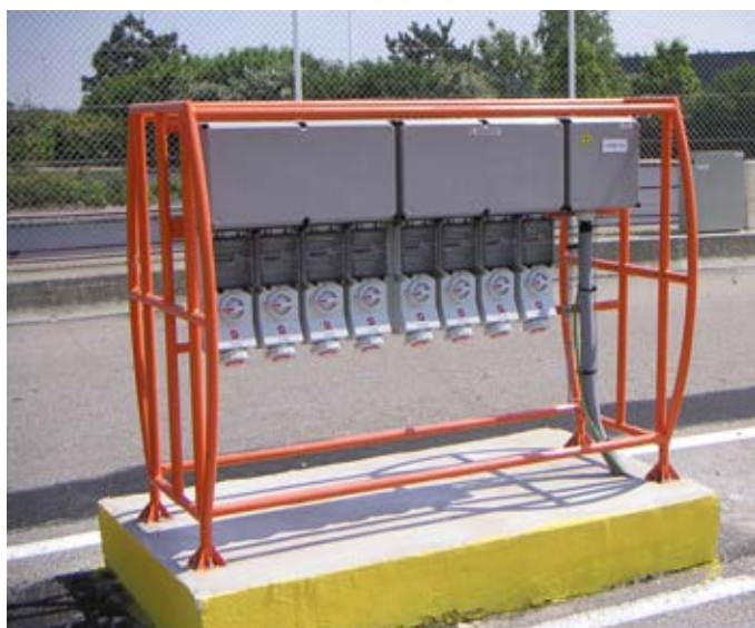
Container Terminal, Le Havre – France
